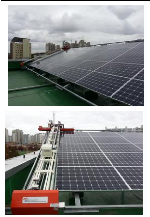
Figure 2: PV panel C&C system installed at the site
