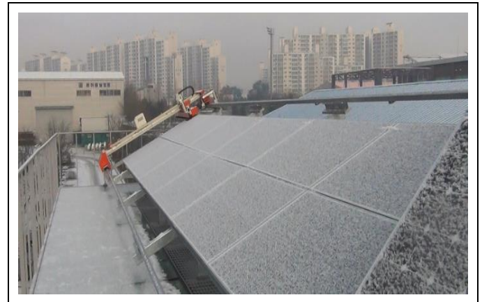
Figure 4: PV panel after snow
